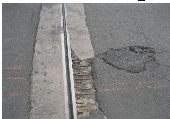
(a) 锚固栓破损开裂
