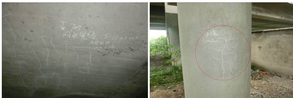
(a) 箱梁内顶板网状裂缝
