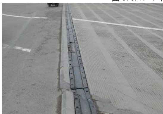
(a) 橡胶板破损
