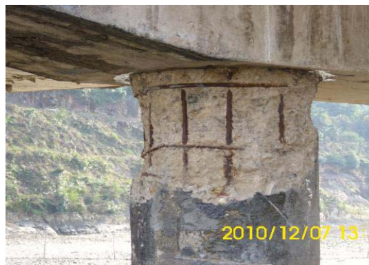
(b) 敲开后钢筋锈蚀
