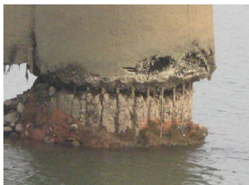
(b) 桩柱接头露筋
