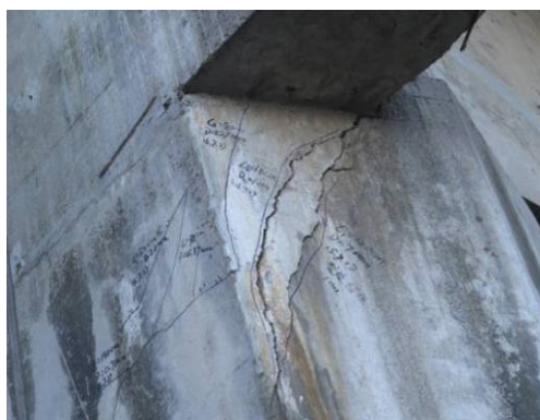
(a) 盖梁侧面斜向劈裂裂缝
