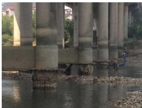
(a) 桩柱接头露筋
