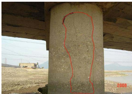
(a) 桥墩立柱竖向裂缝
